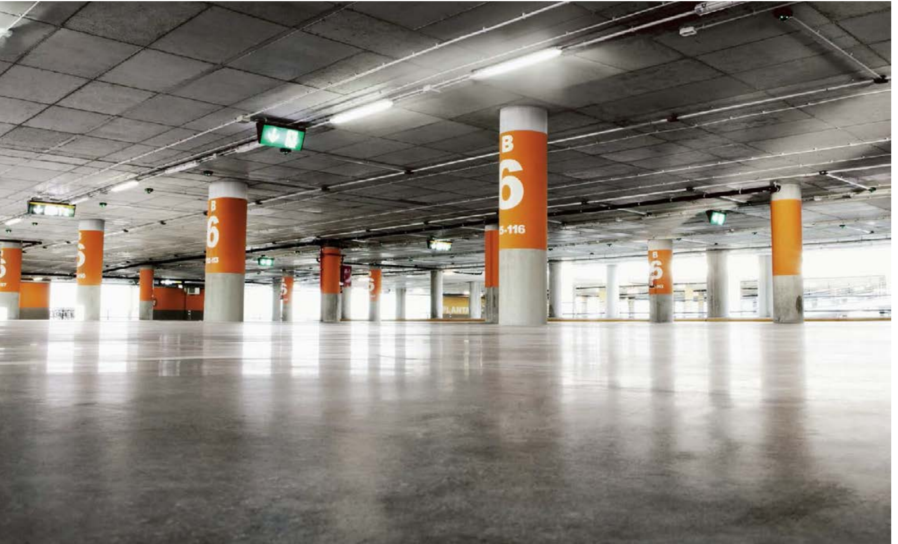
Large-area lighting systems in multi-storey car parks: RS PRO 5800 LED
